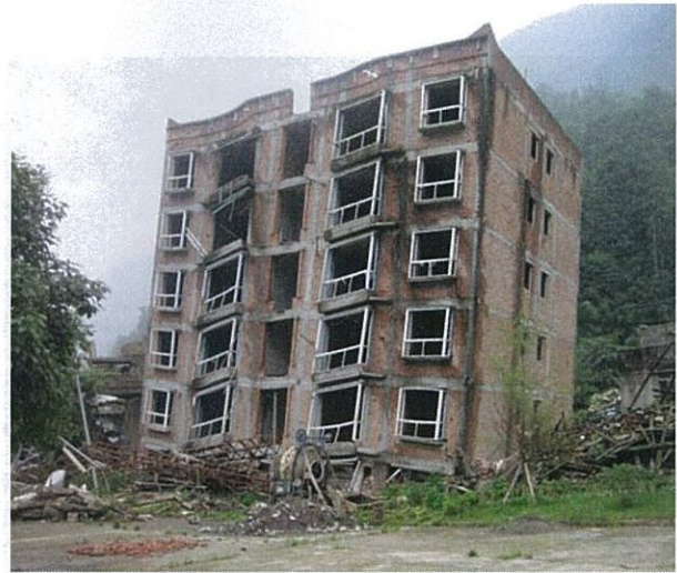
Photo 2: The Damaged Architectures in Beichuan Downtown after the Earthquake
